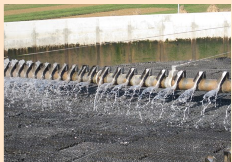
Fig. 2 Trickling filter of Pogradeci WWTP (photo credit by author)
